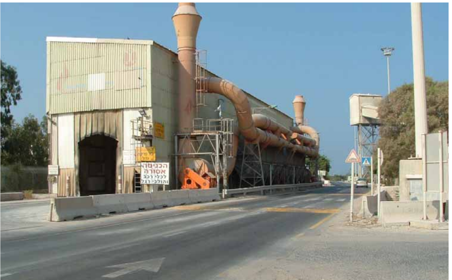
Phosphate Unloading pit Ashdod port 105,000 m 3 /h – Operating Since 1977
