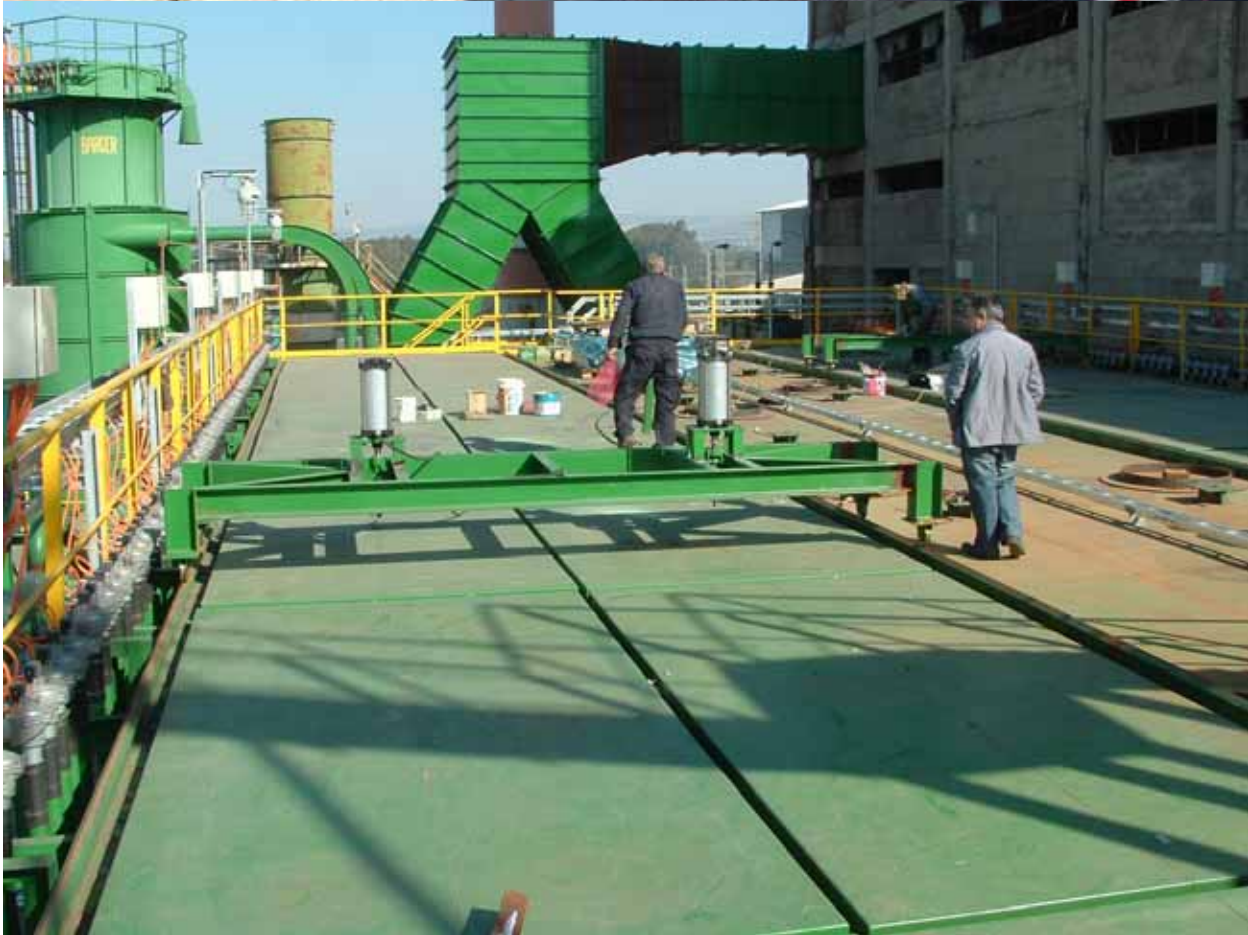
Filter off line type for 60 ton arc furnace 7,016 m 2 filtration area
