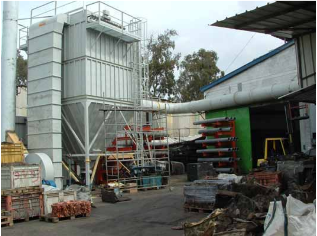
40,000 m 3 /h system for cooper induction furnaces
