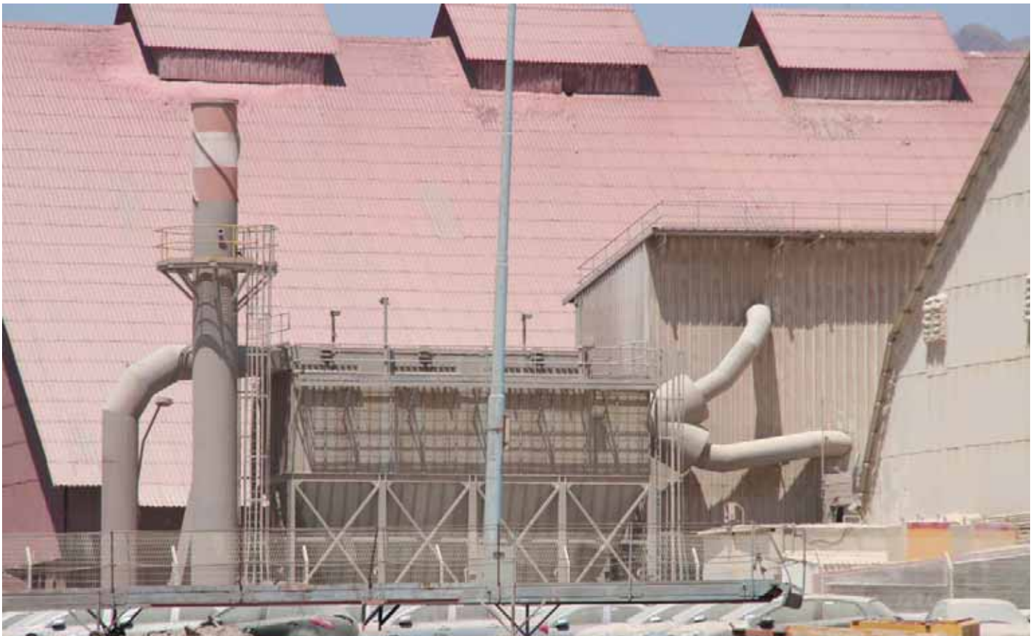
Filter for Phosphate unloading pit Eilat Port 1176 m 2 Filtration area since 1996
