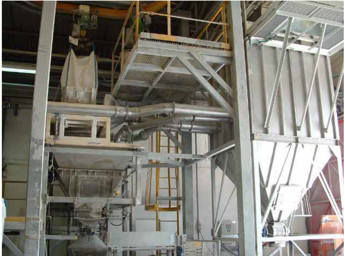
Big Bag discharge system of adipic acid dust made of ss316
