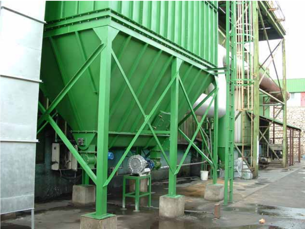
Aluminum Furnace dust and dioxin elimination system 40,000 m 3 /h
