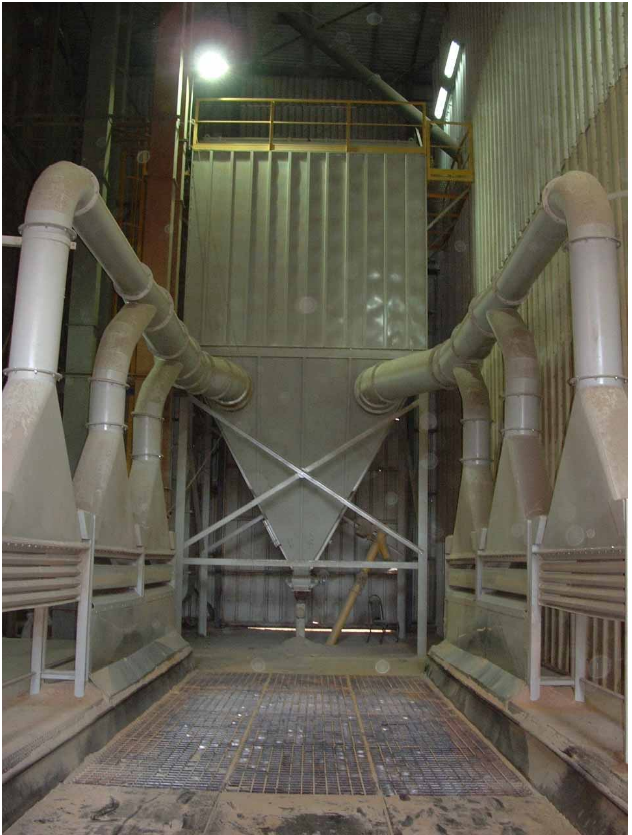
Truck grain unloading pit 65,000 m 3 /h
