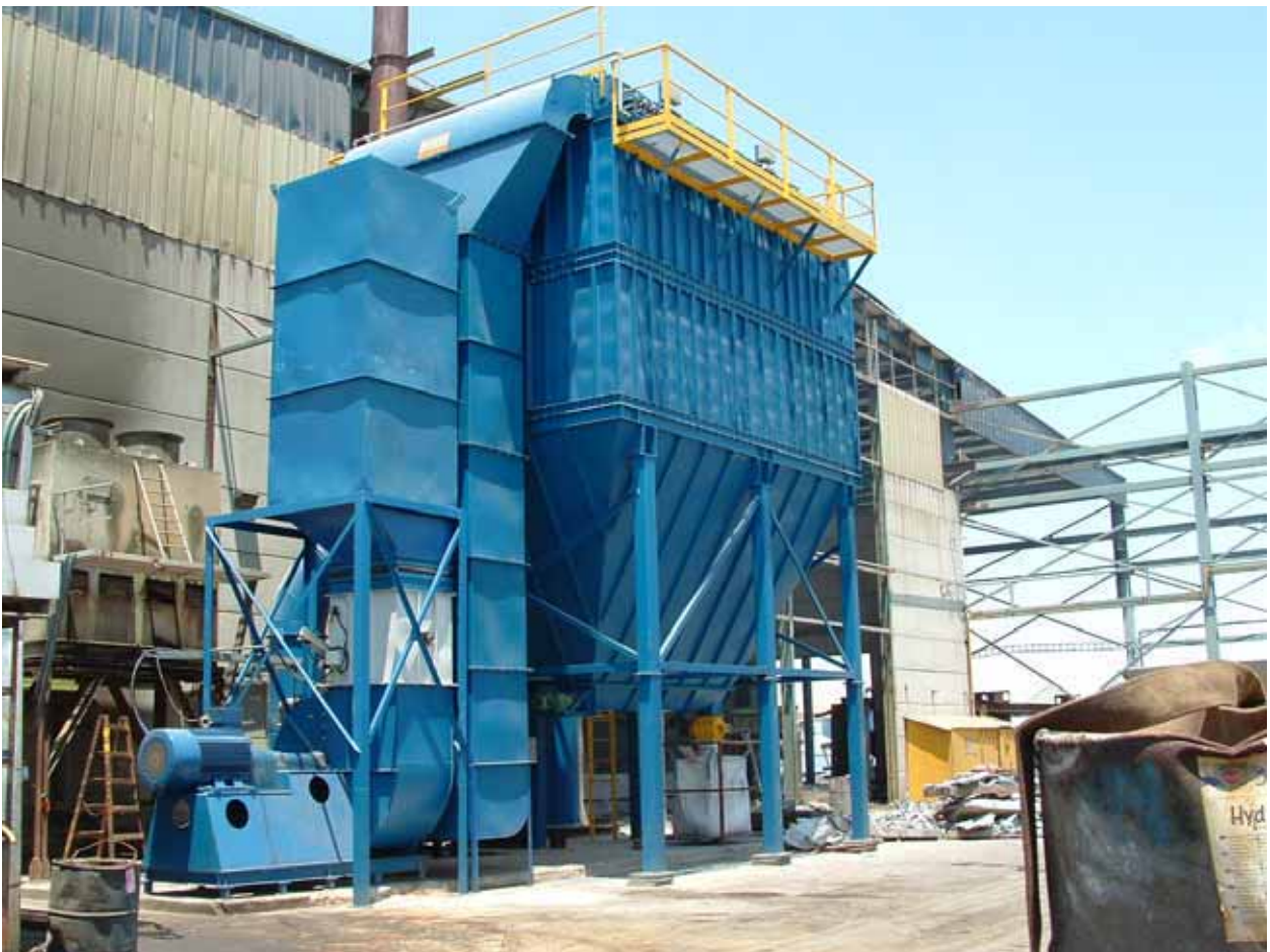
70,000 m 3 /h system for zinc dust from galvanizing bathtub
