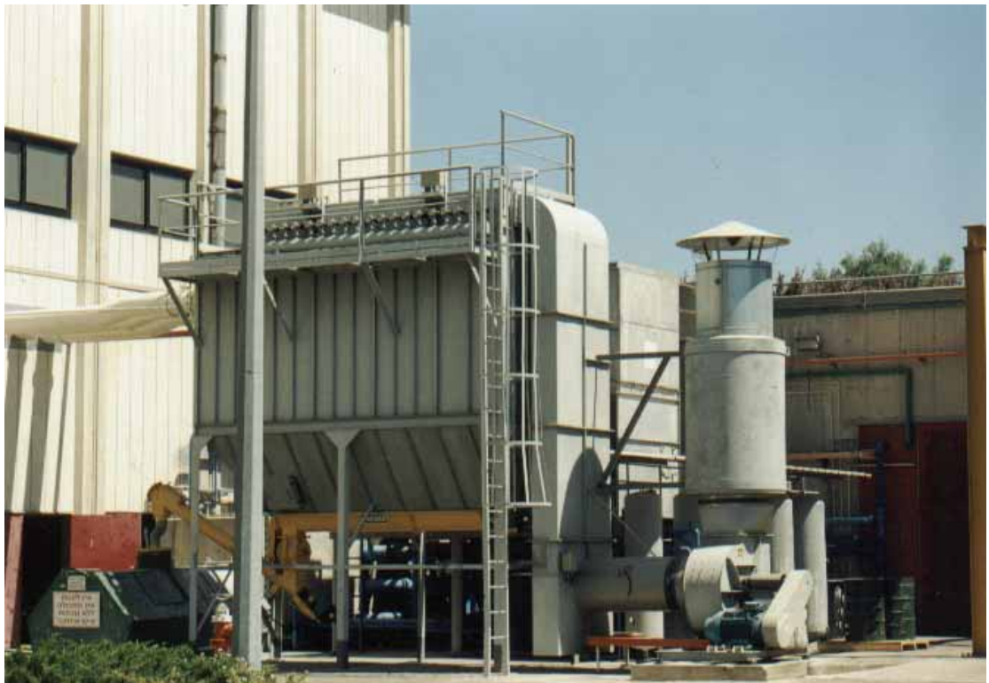
Sand blasting machines dust control
