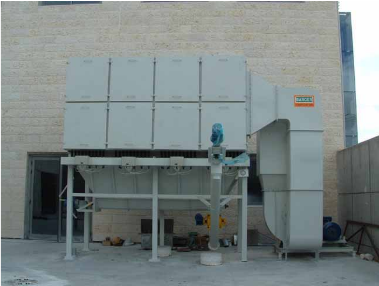
Filter for sand blasting machines using envelope type of filter Bags, side removal, 20,000 m 3 /h installed at ISCAR plant Tefen.
