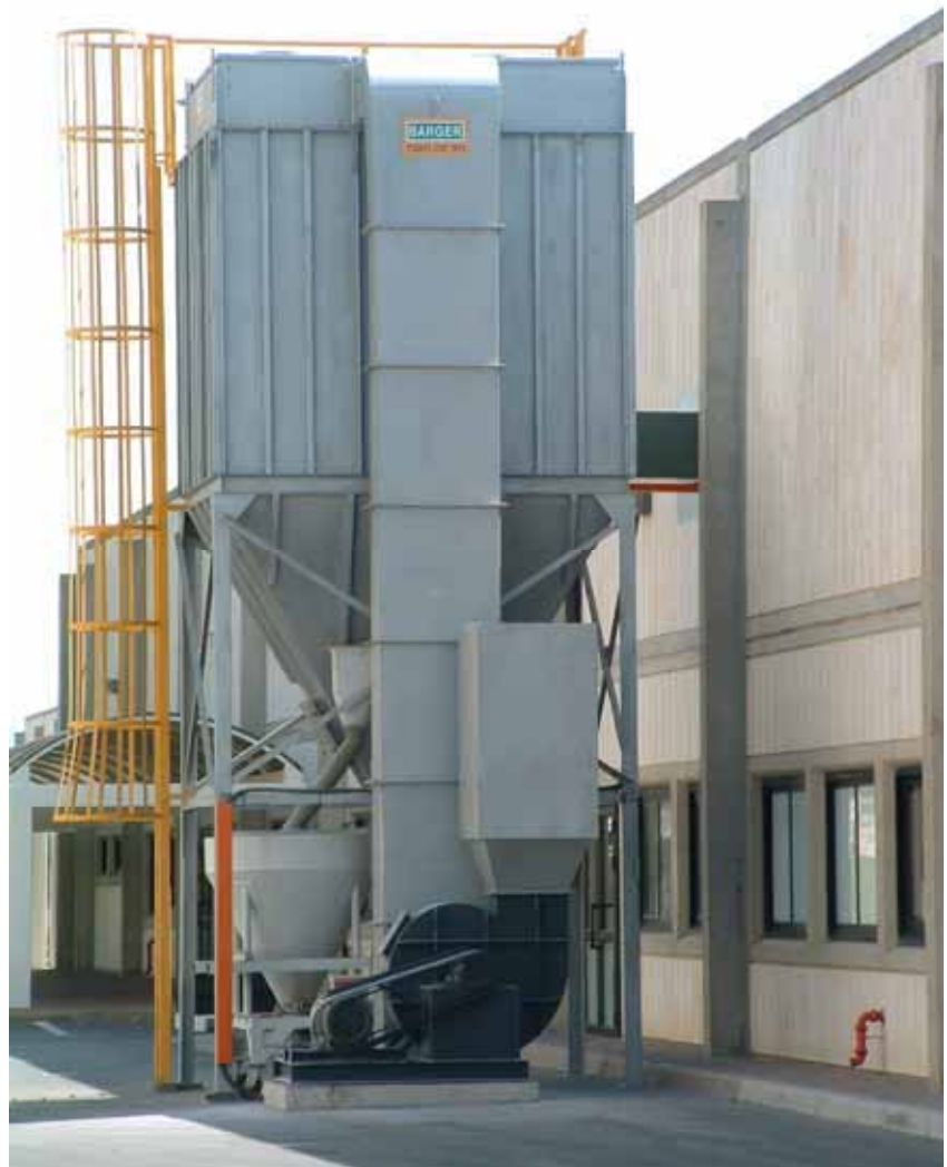
Sand blasting machines system
